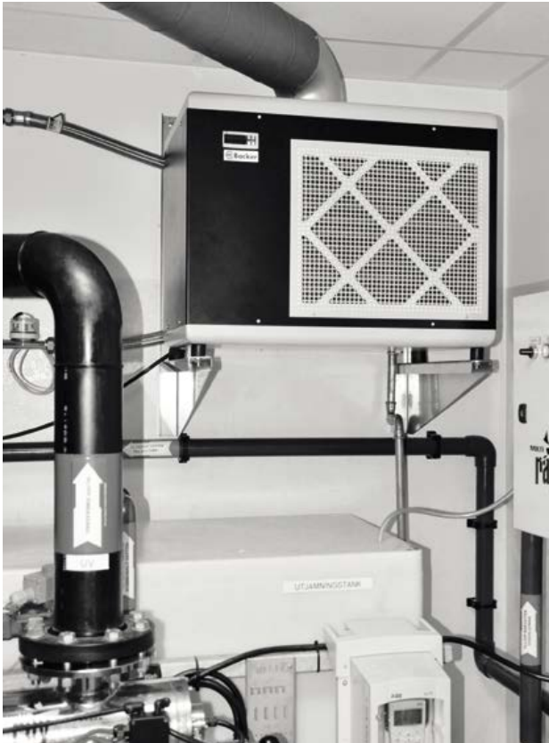
BHP5 installed in a technical room
