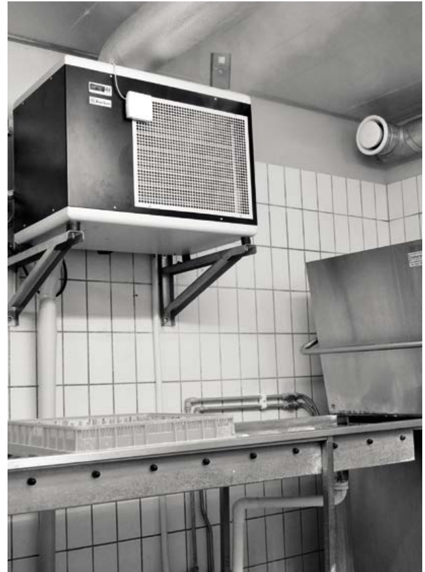
BHP5 installed in a dishwashing room
