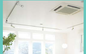
Air Conditioner Units
