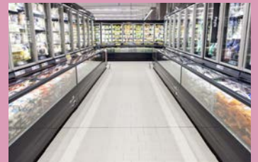
Food cabinet chillers
